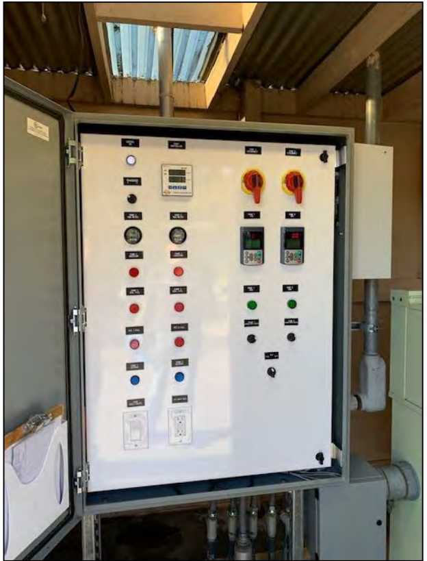
Single to 3 phase electrical upgrade improves motor efficiency at Savory Lift Station
