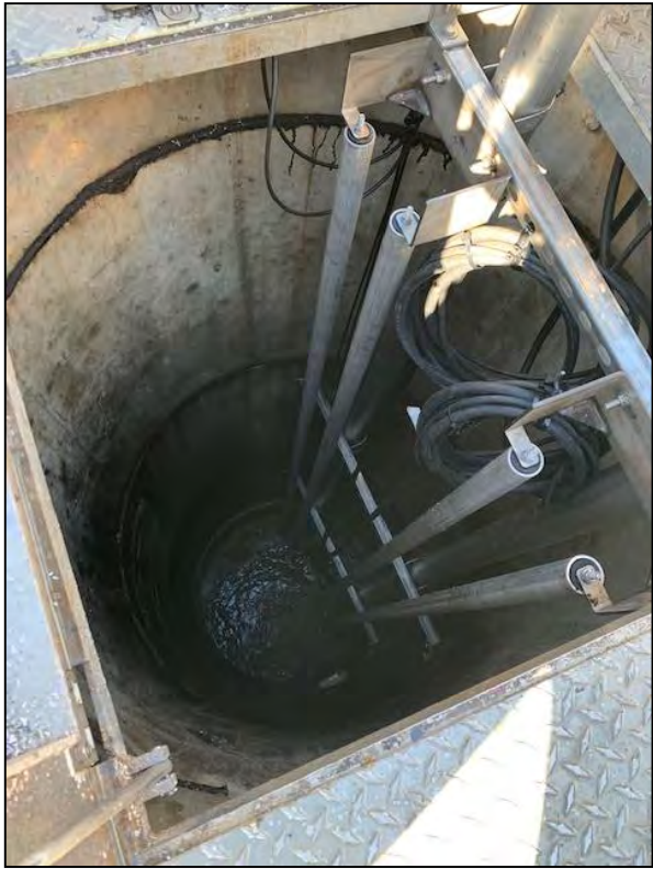
New pump rail system for the grinder pumps
