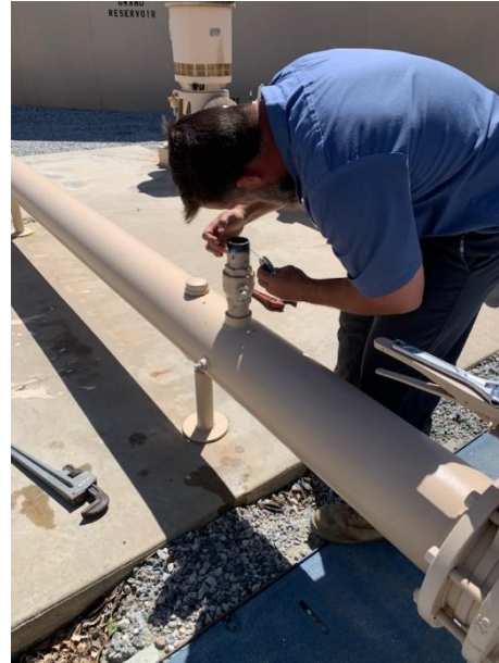
Production Crew installing an new air-vacuum relief valve at the Grand Well
