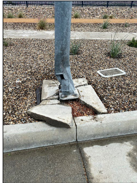
Contractor streetlight crew discovered a hit and run damaged streetlight near the intersection of Esplanade Ave. and Meridian St.
