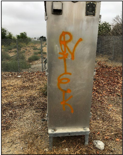
Railroad crossing controller box on Esplanade Ave.
