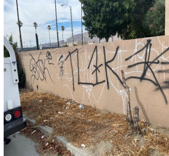
The wall at Tiger Plaza
